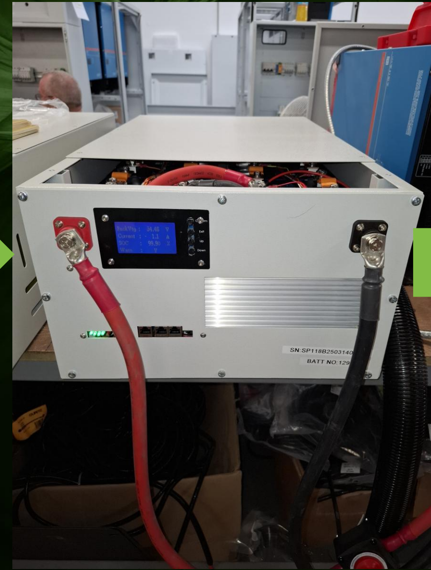
Battery Packs With Battery Management Systems
